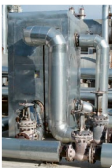
Compabloc condensers at the Rosneft Tuapse refinery
